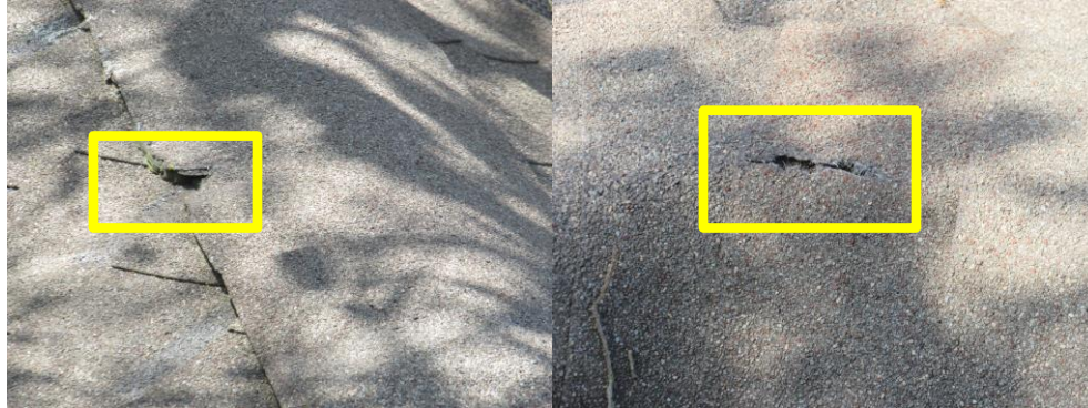
Damaged shingle(s) were noted.
