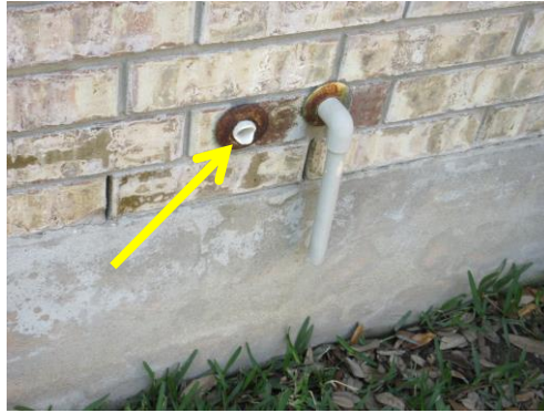
Damaged water heater discharge tube.
