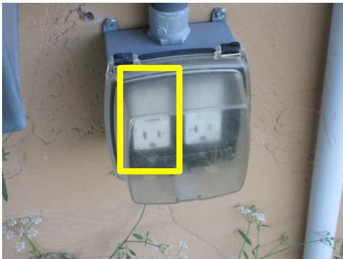
Damaged GFCI protected receptacle located at the main service panels.
