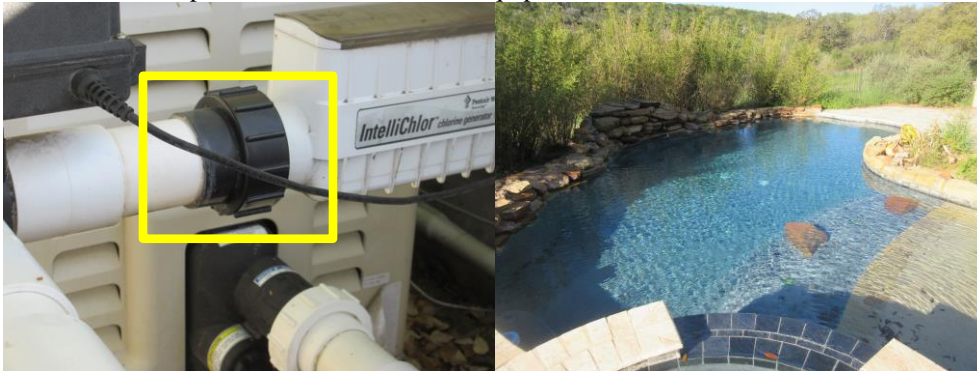
Leaks noted at the pool supply line.
