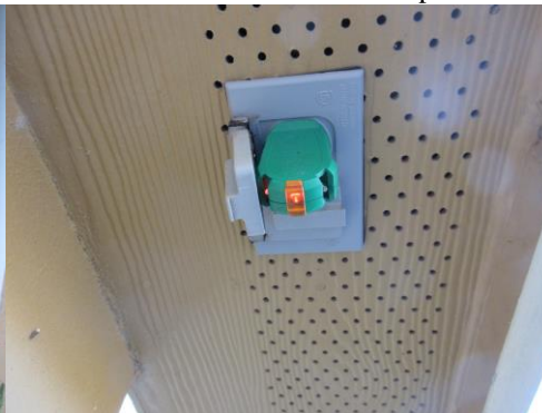
Per current accepted trade practices, all exterior receptacle should be GFCI protected.
