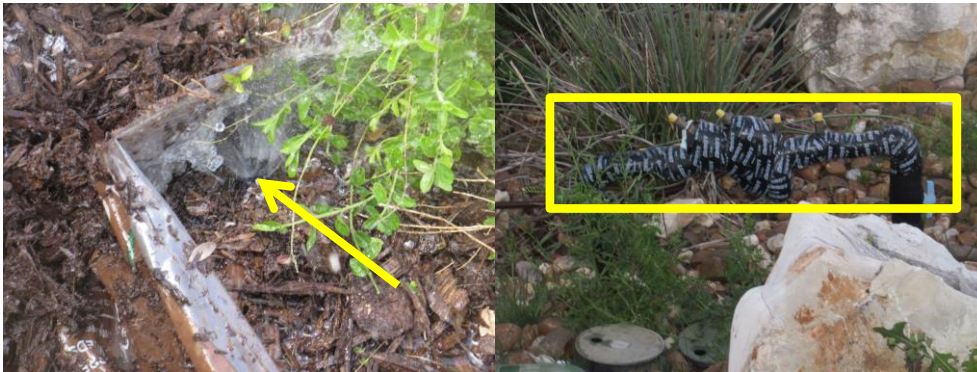
Leak at zone #7 drip system.
