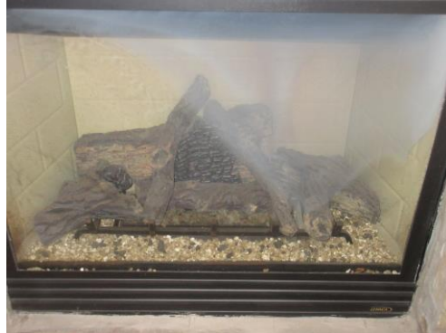
Fogged glass at the Heatilator
