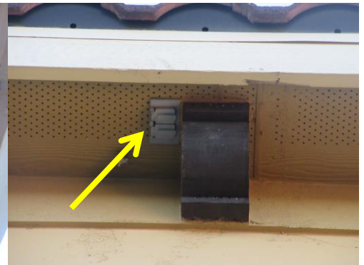
Due to excessive height, various exterior receptacles were not tested and not confirmed for GFCI protection.
