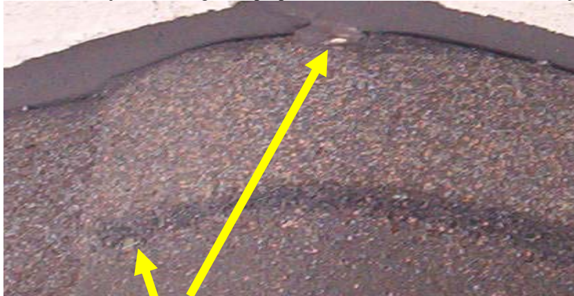
Exposed nail heads that need sealing
