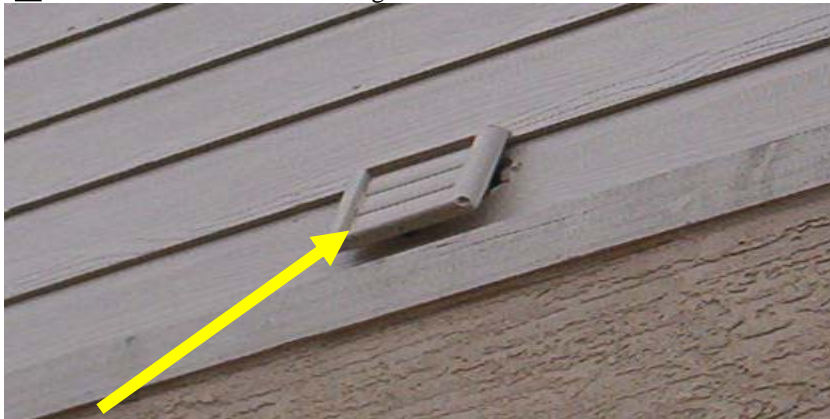
Loose exhaust fan from master bathroom
