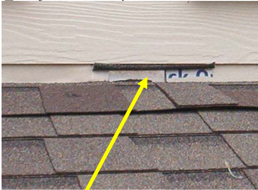
Loose vinyl covering that covers metal flashing, over rear patio
