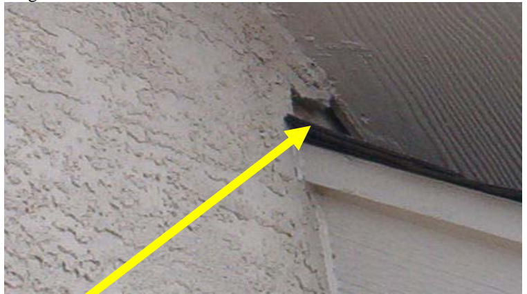
Vulnerable area on the south side upper level
