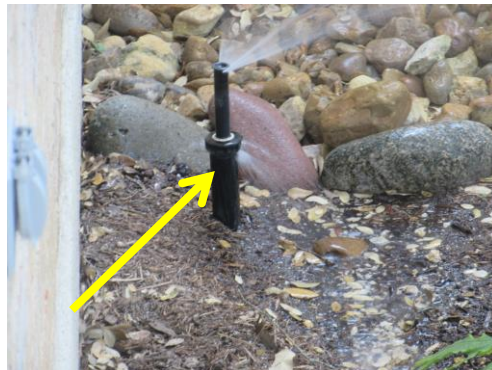
Damaged spray head at zone #2.
