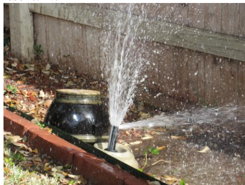
Malfunctioning sprinkler heads at zone #1 and zone #4
