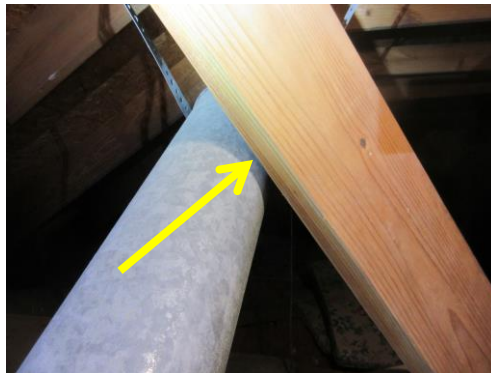
The furnace exhaust flue is too close to combustibles.
