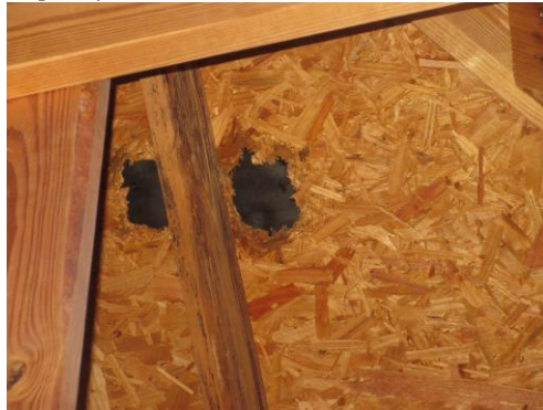
Damaged roof decking noted.
