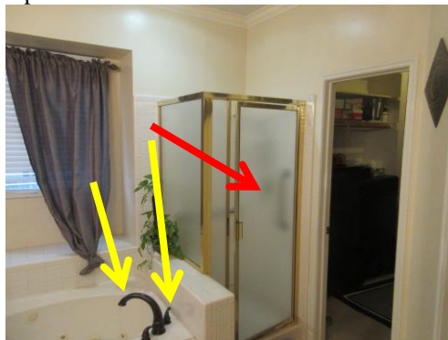
Loose faucet and hot water handle at the master bathroom tub. (yellow arrows)
